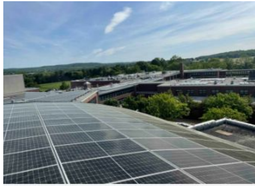
Solar Panels on Roof of North Hunterdon HS
